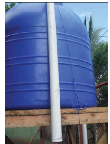
FIRST-FLUSH PIPE FOR THE TANK PROVIDING WATER TO THE KITCHEN.
